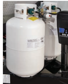
30# LP Tanks with Cover
