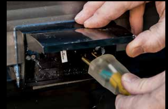
Convenient Outside GFCI Protected and Covered Outlet.
