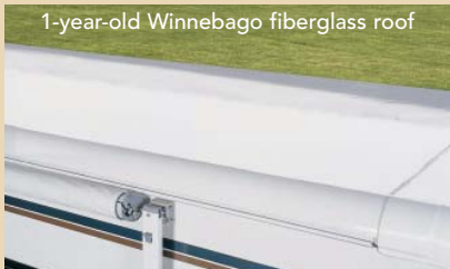
1-year-old Winnebago fiberglass roof
