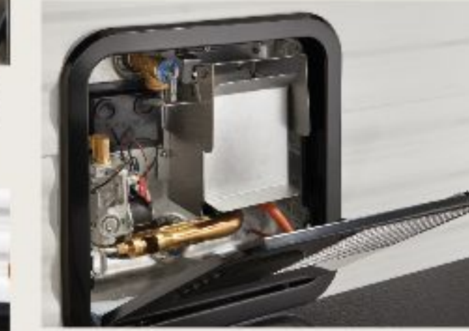
Six gallon direct start ignition (DSI) water heater
