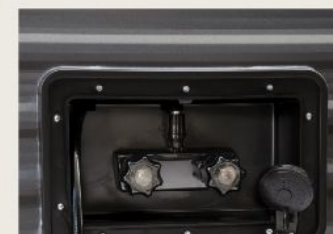
Hot and cold outside shower reduces tracking dirt indoors
