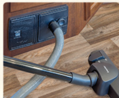
CENTRAL VACUUM SYSTEM
