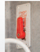
Hot water bypass valve
