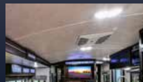
Dual Ducted A/C System
