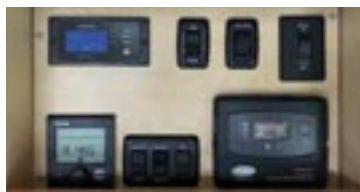
Convenient control center monitors capacities
