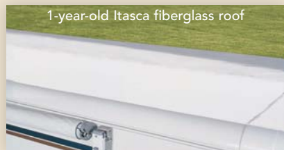
1-year-old Itasca fiberglass roof
