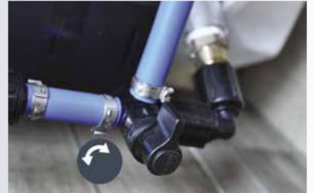
Water heater bypass & winterizing valves make draining the system for winter storage a breeze.
