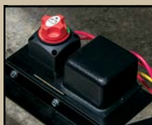
Handy exterior battery disconnect.
