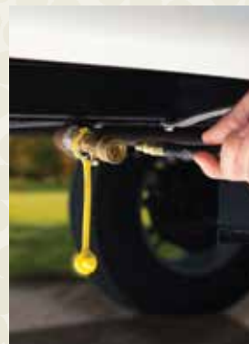
LP gas hook up
