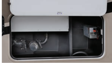
Heated/enclosed holding tanks use warm air from the furnace to protect tanks and valves. (N/A 2251SLE, 2551DSLE, MBS and Transit)
