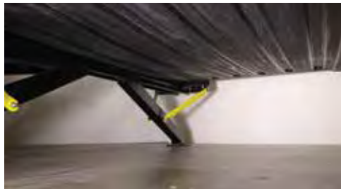
Heat is routed into individually insulated holding tanks to keep them, the valves and PEX lines warm.
