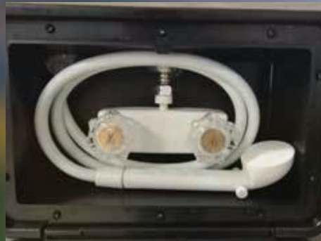
Outside Shower With Hot And Cold Water
