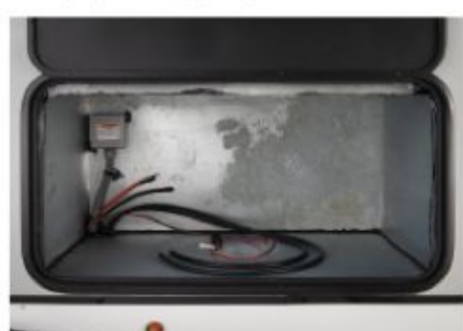
Generator Prep (Standard 27KB, 29SS)
