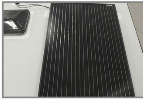
SOLAR PANEL ON ROOF
