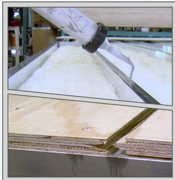
GLUED & SCREWED PLYWOOD FLOORING 5/8" Tongue & Groove Plywood Floors Glued & Screwed on Aluminum Floor Joist (16" on Center)
