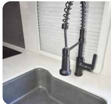
Residential faucet fixtures.
