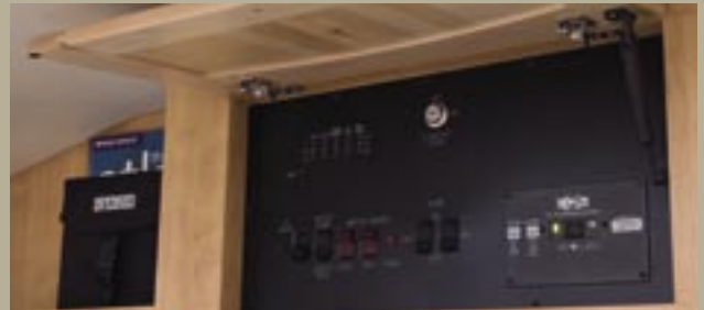
An electronic control panel is conveniently located above the entry door.
