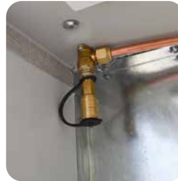
Exterior Propane Connection
