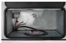
Generator Prep (Standard 27 KB, 29 SS)
