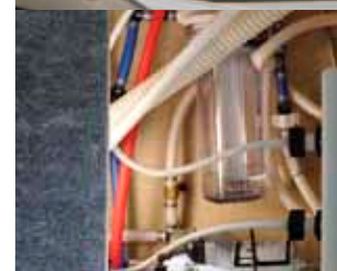
Outside Antifreeze Inlet with Easy Access Water Pump in Storage Compartment for Convenient Winterizing (Std. Signature FW)
